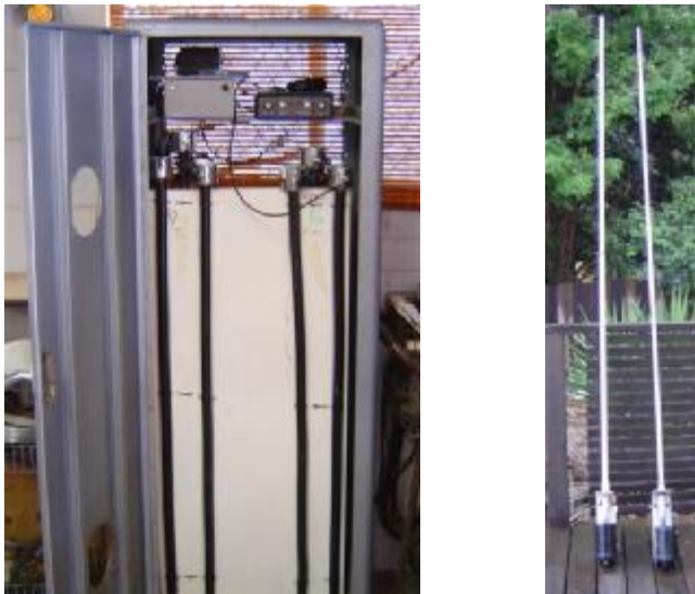
Fig.1 6 m radio cabinet and finished Rx and TX antennas
